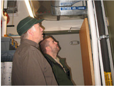
Facilities maintenance specialist Dick Logan (left) and forester/ranger Shawn Jones, stationed in Woodruff, look over pipes and duct work that make up the new geothermal unit. The unit provides warmth in the winter and cooling in the summer WDNR Photo
