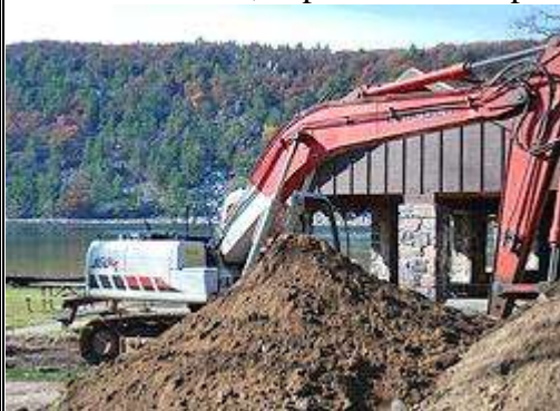
Scenic Devil’s Lake bluff served as a backdrop to reconstruction of the bottom withdrawal pipe.
