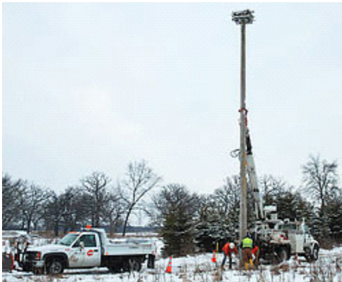
The WE Energies crew took about an hour to erect the 50-foot pole and osprey platform. WDNR Photo
