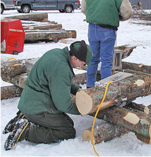
A member of the crew lashes logs together to construct a fish crib. WDNR Photo
