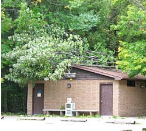
A large tree caused damage to this shower building at Potawatomi State Park. WDNR Photo
